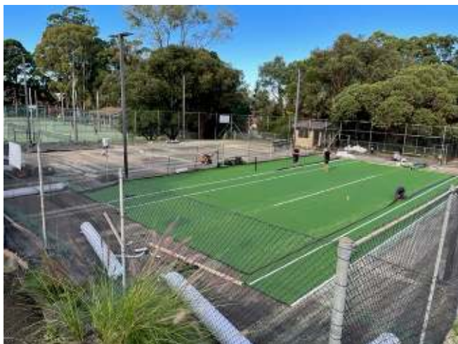
Figure 2. In 2022 Voyager is investing in resurfacing 16 tennis courts, installing new lights over 19 courts, upgrading fencing and refurbishing 6 tennis clubhouses.
